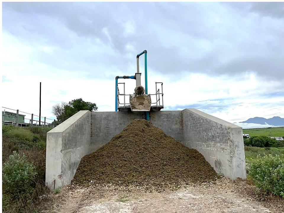
Part of a mechanical separator system with the separated solids.
