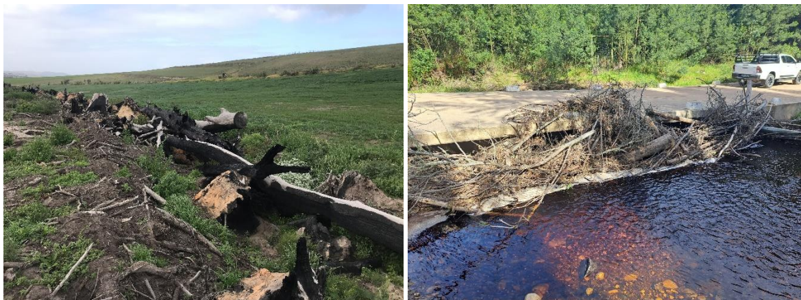
Figure 16. Photos showing burnt alien trees pushed into a wetland (left) and a culvert blocked by slashed alien vegetation discarded in the river upstream.
