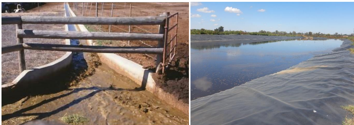
Figure 15. Slurry transferred from wash down areas via a concrete channel (Photo credit ARC), and a slurry dam with plastic liner (Free State).
